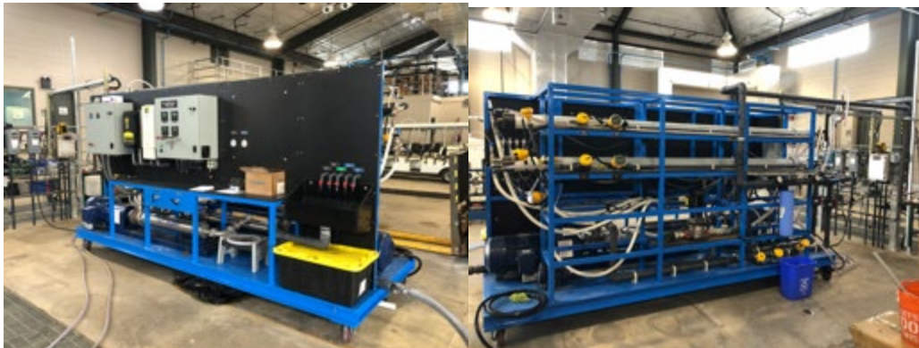
Figure 4. Reverse osmosis treatment system at BGNDRF.
