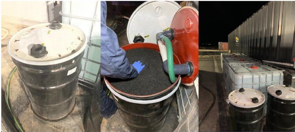
Figure F. Activated Carbon System
