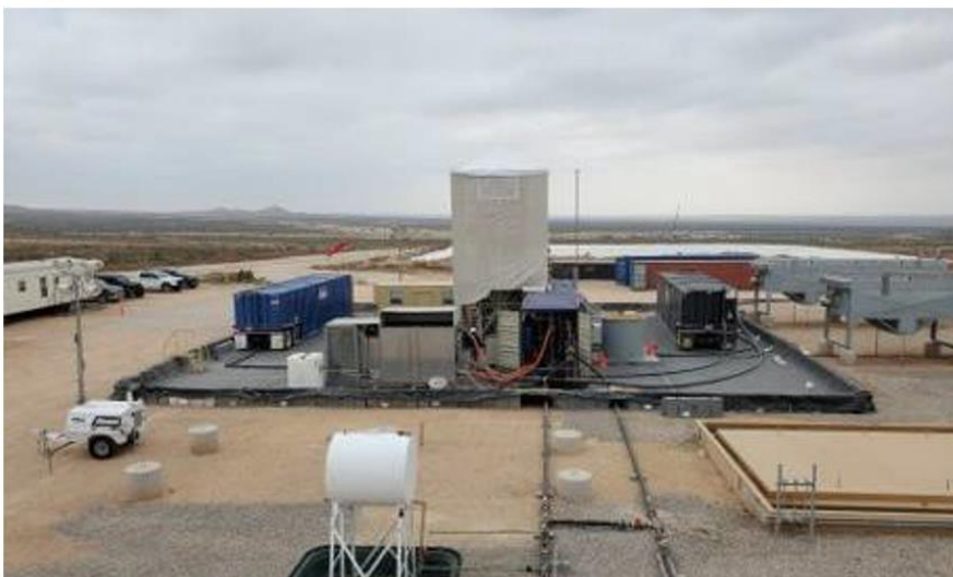
Figure C. D1 at the Pilot Location with Feed Tank (black tank) and Fresh Water Tank (blue tank)
