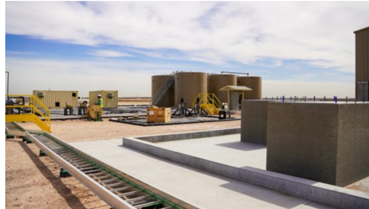
Large Storage Tanks
