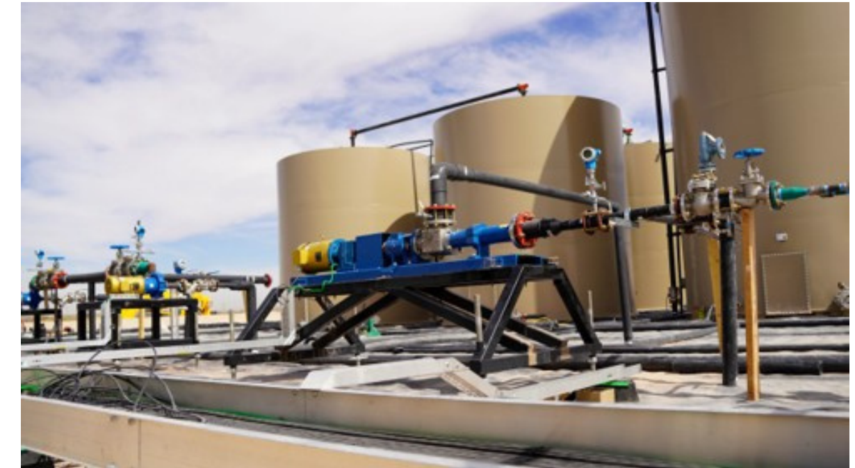
Process Piping & Valves
